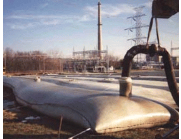
Figure 22. Geotextile tubes can be used to store and dewater hydraulically dredged sediments.
