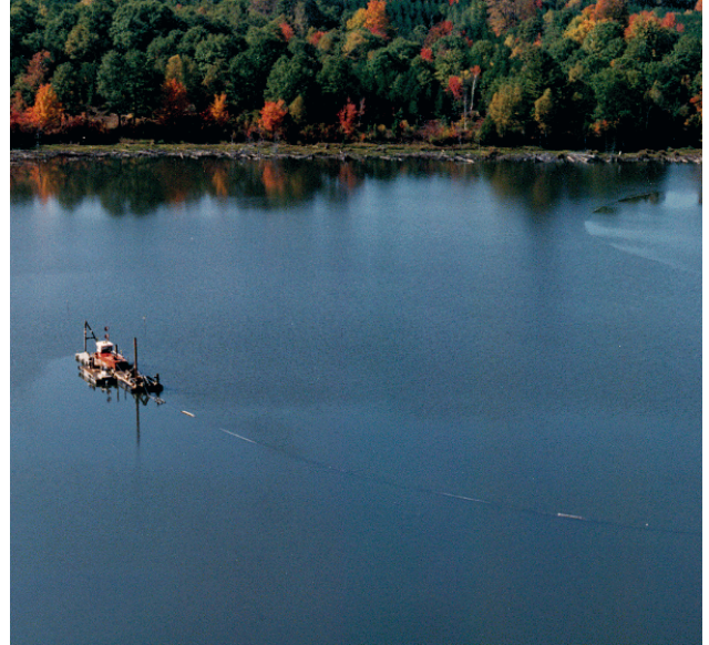
Figure 20. Hydraulic dredging. The floating pipeline is visible behind the barge at the bottom of the photograph.
